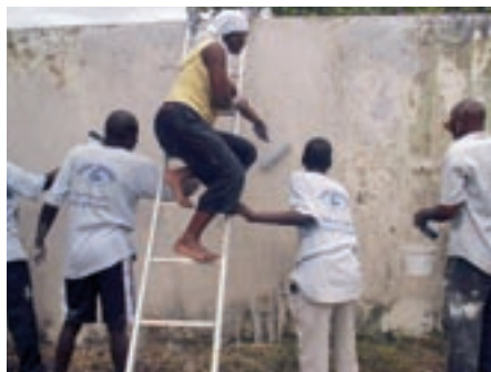
The whole team came in on a Saturday to paint the perimeter wall. Activities outside work help build team spirit. KENYA
