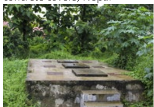
Figure 3 Protected pits with concrete covers, Nepal
